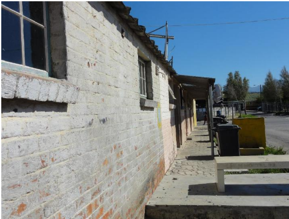
Fig 5. Hostel 33 as part of a group of houses within Lwandle. This formed part of the Hostel to Homes project whereby hostels were converted into family houses.
