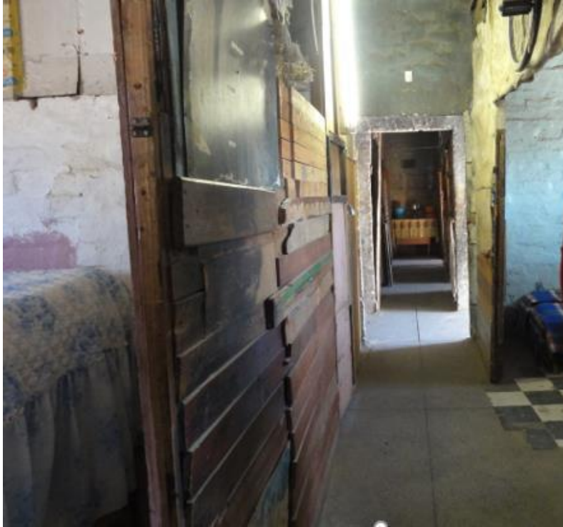
Fig 6. Hostel 33 looking down the full length of the passage created by the further division of the interior spaces into rooms
